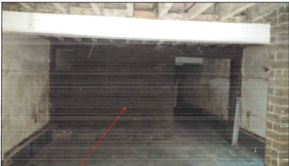
Photograph 2 – View of basement, facing east. Concrete slab appears not to be compromised.
